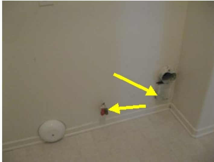
Laundry Dryer Vent
