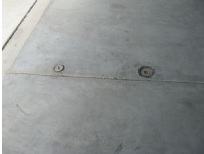
Garage Flooring Condition
