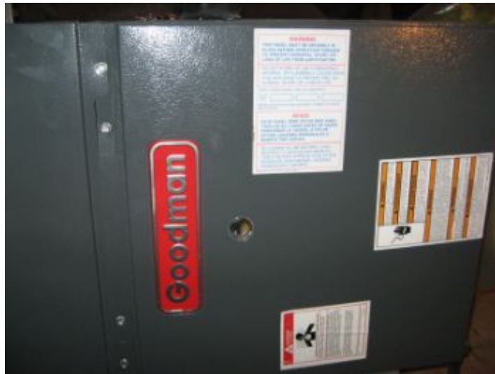
Heat/AC Heater Condition
