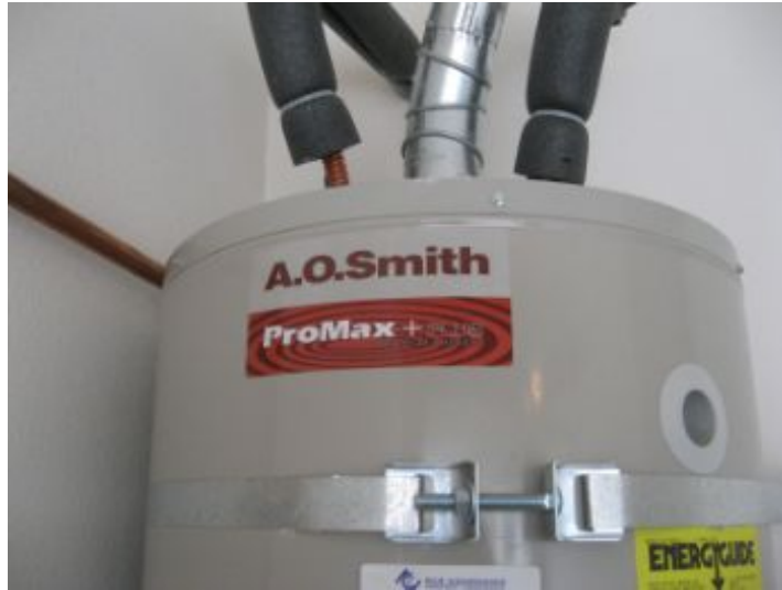
Water Heater Water Heater Condition
