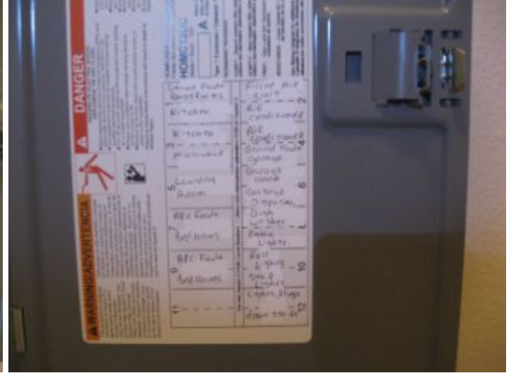
Electrical Electrical Panel
