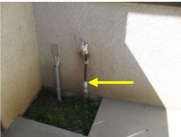
Grounds Water Shut-off Valve Condition
