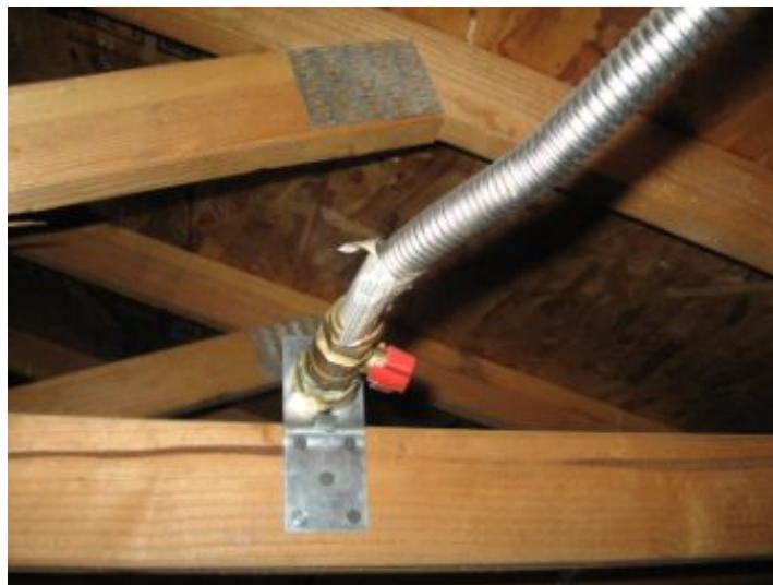
Heat/AC Gas Valves
