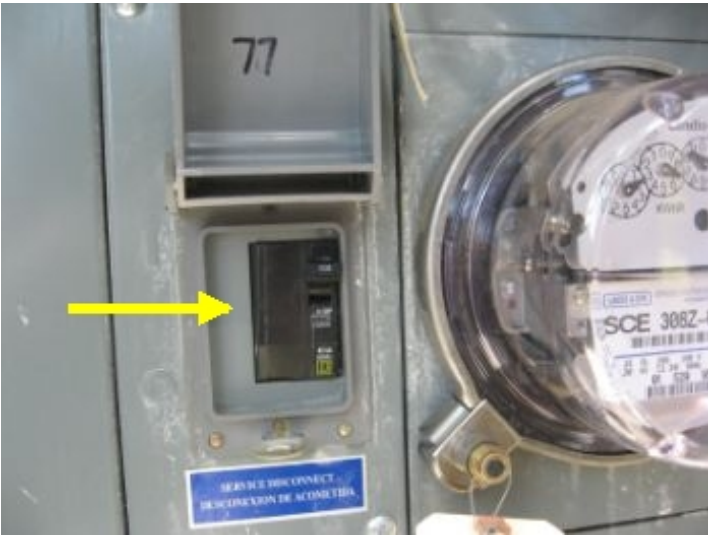
Electrical Main Amp Breaker
