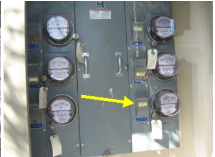
Electrical Main Amp Breaker
