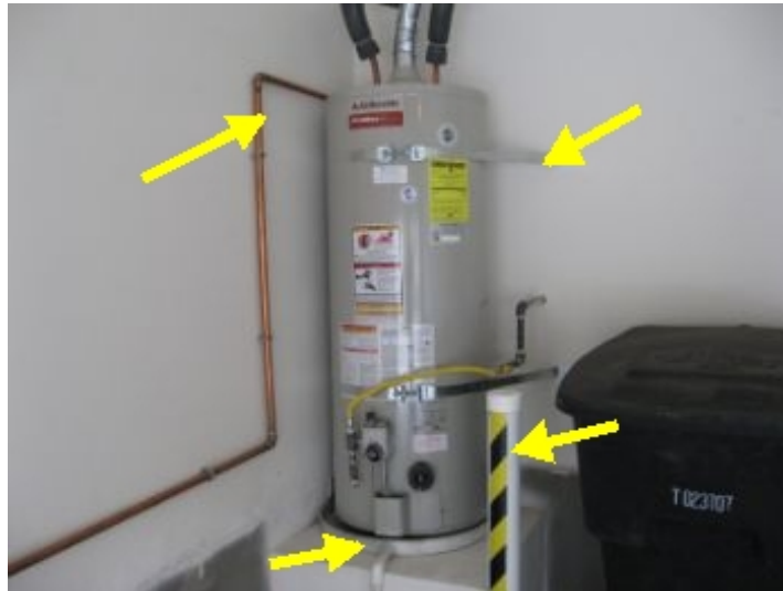
Water Heater Strapping
