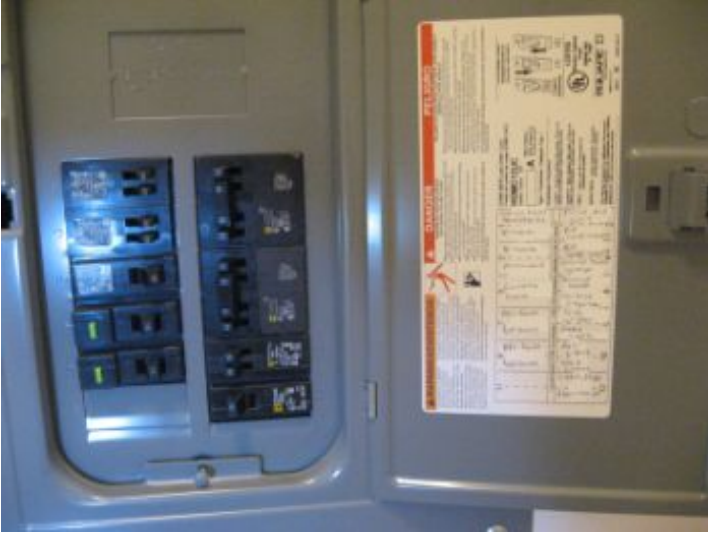
Electrical Electrical Panel
