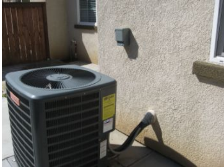
Heat/AC AC Compress Condition
