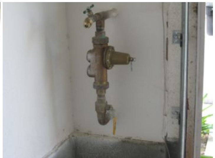
Grounds Water Shut-off Valve Condition
